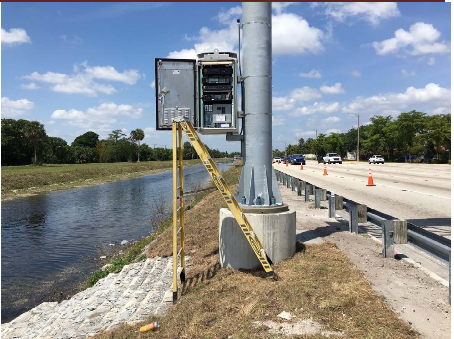
Figure 1; Cabinet Height at DMS 1
