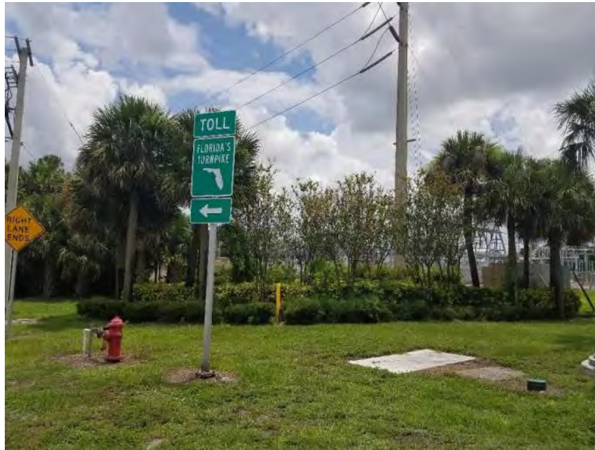
Site 65 - Turnpike Substation Northeast looking southwest
