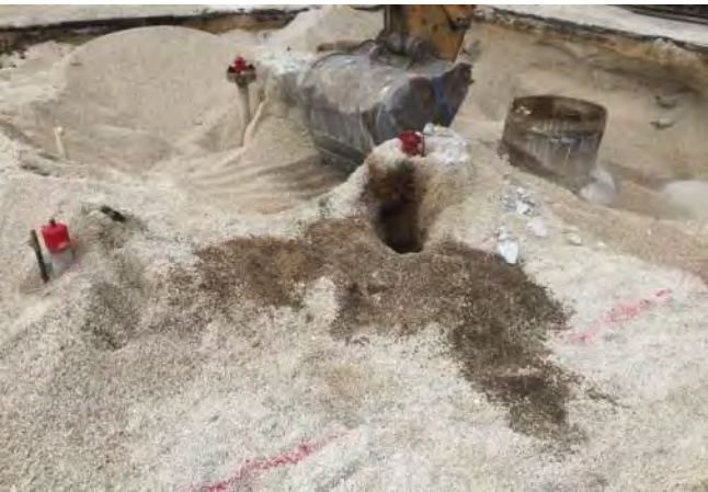
Gas Fill Port with Stained Soil, No Odor Looking SW
