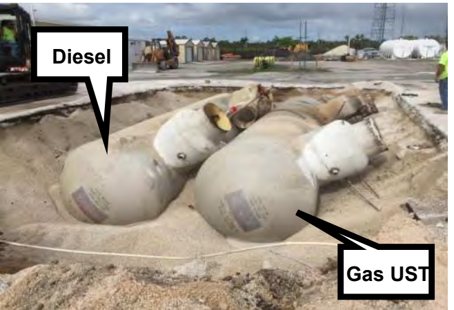
Diesel Gas UST USTs Floated to Top of Excavation Intact Looking West
