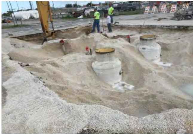
2 10,000-gal Double-walled Fiberglass USTs Looking to the NE
