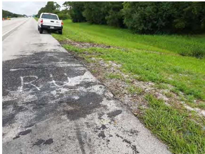
Site 58 – Spill (Station 1285), east side of northbound lane South looking north
