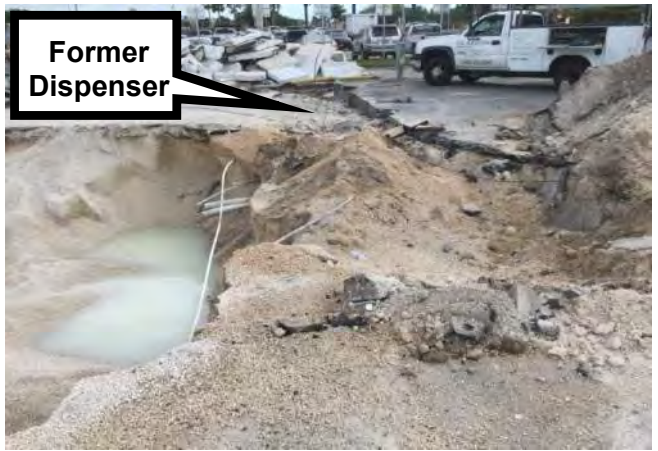
Former Dispenser Former Dispenser Island; E End of Tank Field Looking to the NE
