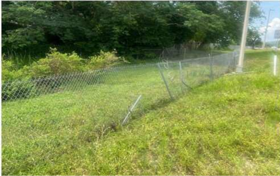
Figure 3: Undesirable Fence Condition - Damaged Fence Post
