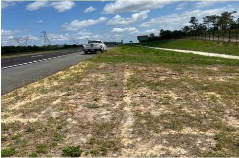
Figure 11: Undesirable Turf Condition - Front Slope
