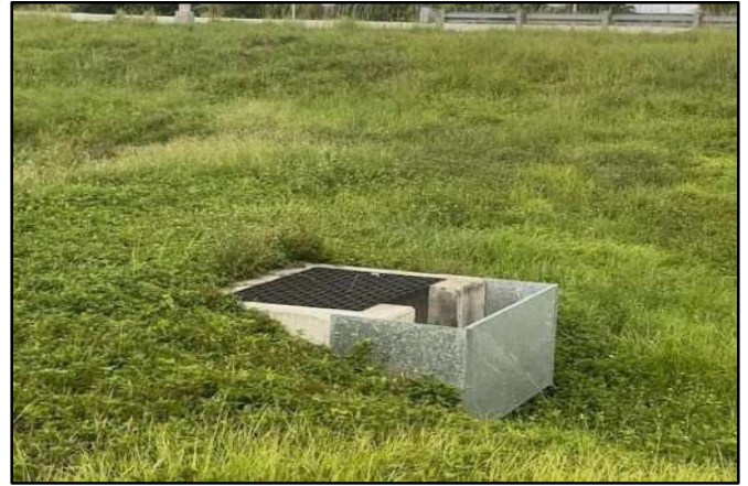
Figure 12: Inlet with Skimmer
