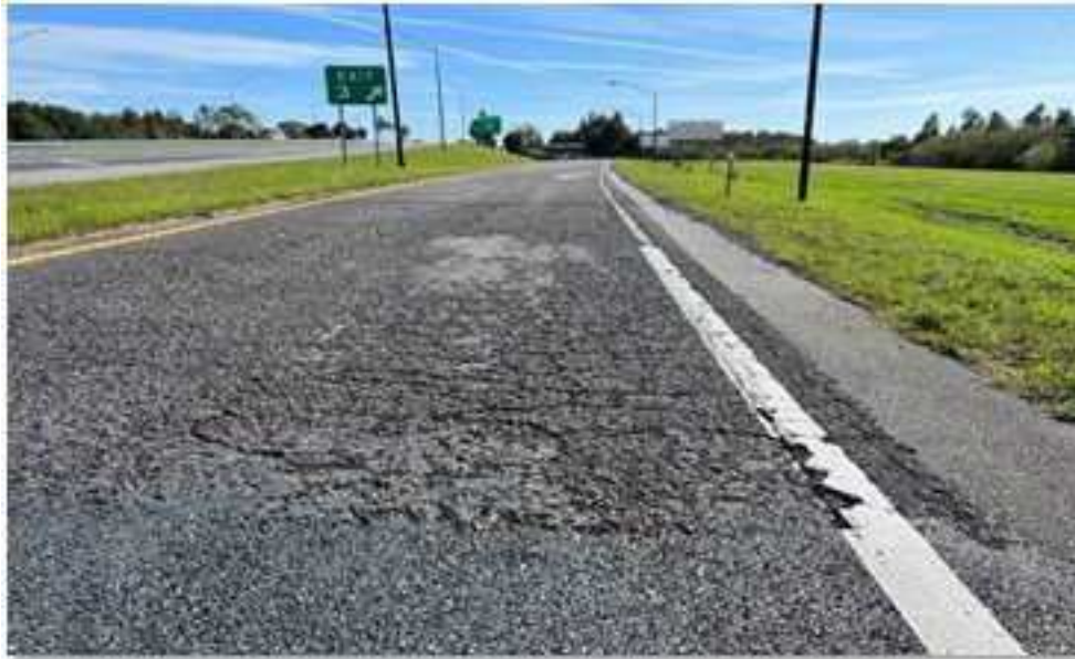
Figure 1: Undesirable Pavement Condition - Class III Cracking
