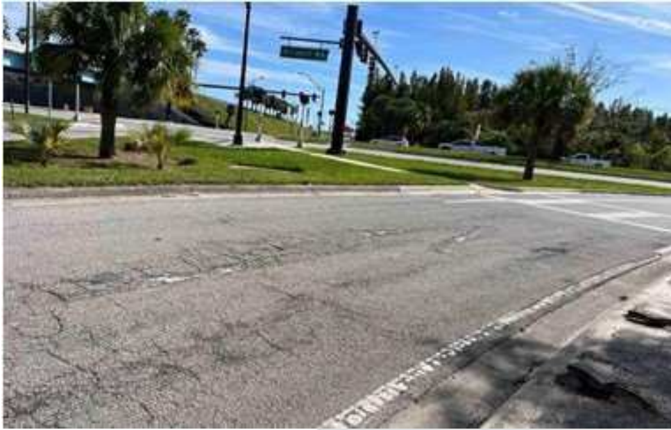
Figure 7: Undesirable Pavement Symbol / Cracking
