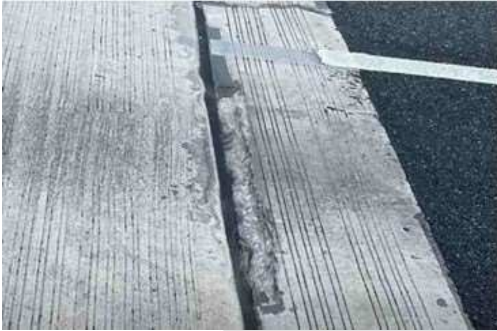
Figure 5: Undesirable Joint Condition
