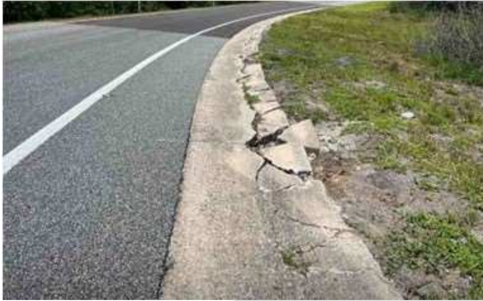
Figure 9: Undesirable Shoulder Gutter
