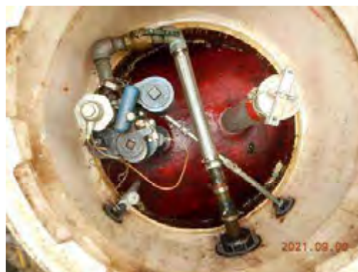
2021-09-08 Diesel STP sump
